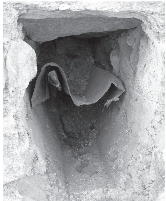
Figure 12.8. Primary roof scupper, or drain, unblocked in the northern bay of the east elevation in 2008, showing lead lining over disintegrating timber channel (Photo: Roland Harris).
